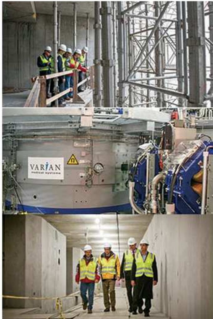
In the space currently filled with scaffolding (top), the Proton Therapy Center's massive gantries will aim
